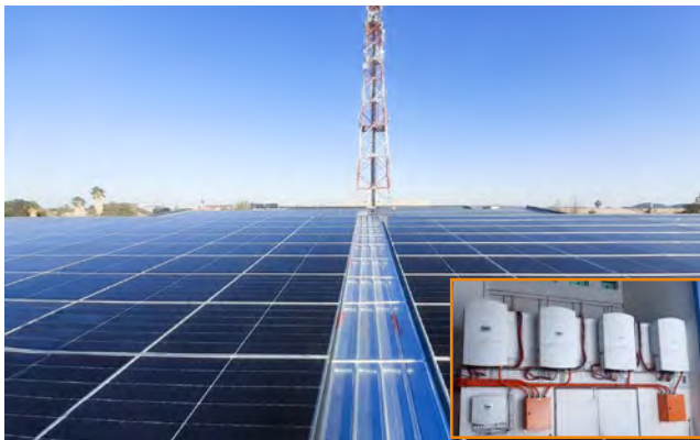
SolWorx Project, Namibia 272kW
