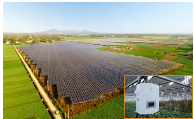
Hubei Guanyin Agricultural-photovoltaic hybrid PV plant 20MW
