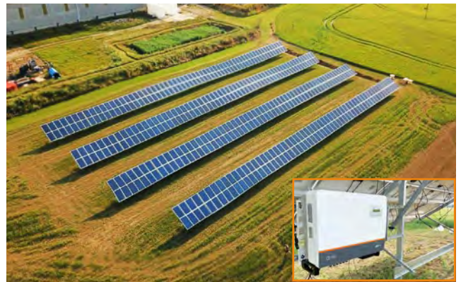
Lincolnshire, UK 140kW
