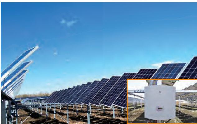
Hebei Zhangbei Agricultural-photovoltaic hybrid PV plant 50MW
