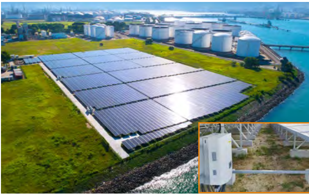
JTC Solar Farm, Singapore 5MW
