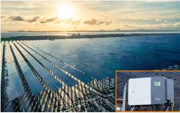
Zhejiang Ningbo Tidal Flat Project 300MW
